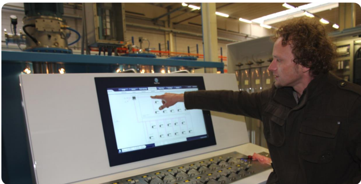
Herman Bouman shows that PROCENTEC ComBricks allows for remote monitoring of the PROFIBUS installation from a safe zone.
